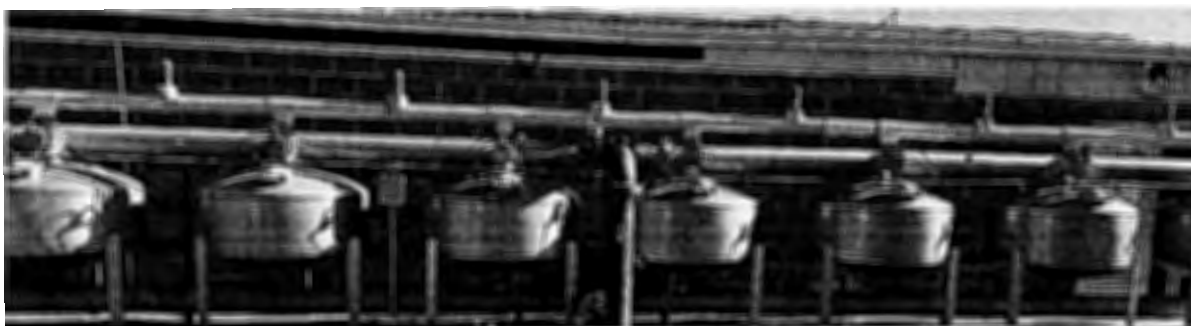
View of the existing Sand Filters
