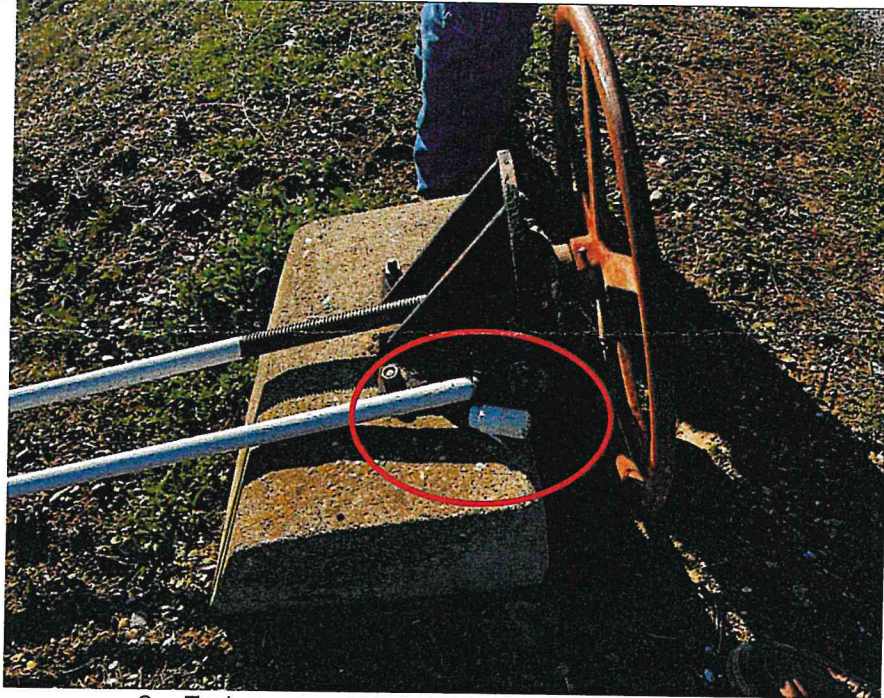
2. End cap repair required at outlet vent pipe.
