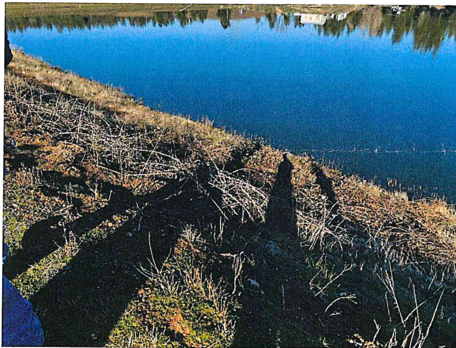
5. Continued vegetation control of berry vine brush required on the upstream face of East Dike.
